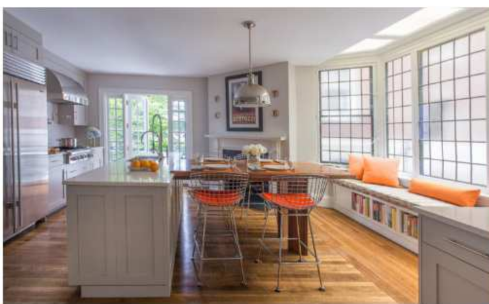
The original quartersawn oak flooring was carefully torn up when the kitchen was gutted. The wood was relaid and stained to blend in with the additional planks needed to accommodate the new layout. —Photo by Eric Roth/Design by Renovation Planning
